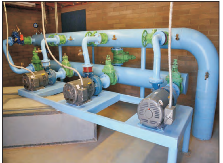
Industrial Pump Systems
