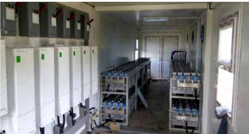
Interior view of solar powered container built with a modular system of battery-based inverters and charge controllers
