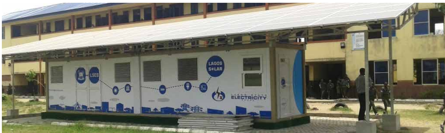
Full exterior view of solar and storage solution for schools and PHC's throughout Lagos State, Nigeria
